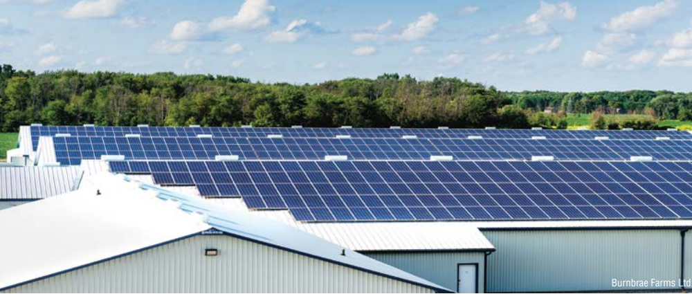
Solar panels on an egg barn
